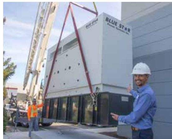
Photo: Director of Programs, Billy Bartz, guiding the diesel generator into its new home just outside the REFB warehouse on Brickway Boulevard.
